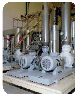
Pumps, compressors, fans
